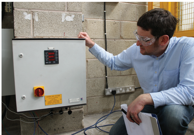
Pumpflow's Engineering Manager Sean Whiston with one of the panels designed by Endress+Hauser
