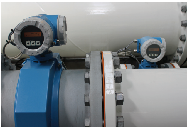
Two of three Endress+Hauser Proline Promag flowmeters installed on the test bed
