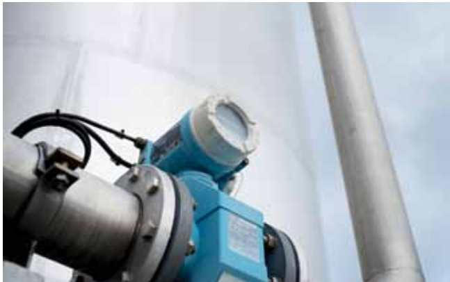
Industrial water treatment and wastewater treatment
