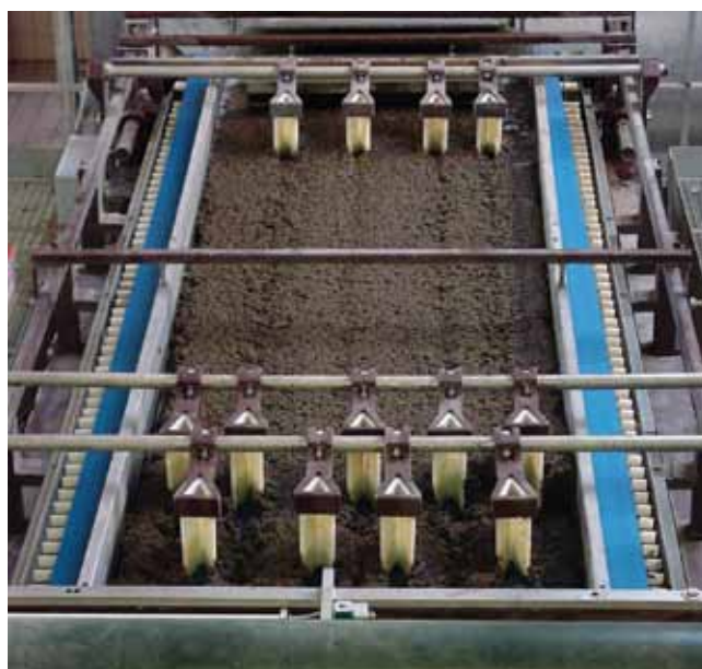
Belt filter in a sewage facility for sludge dewatering
