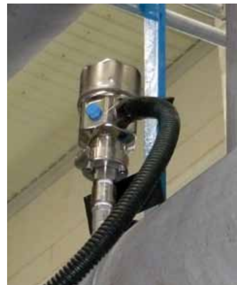
Accurate pressure measurement in a membrane system
