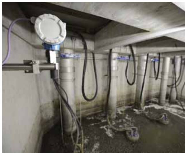
Dependable level measurement in the extensive sewerage system
