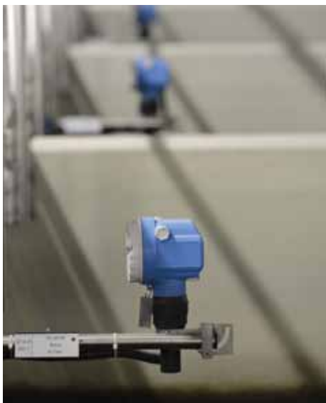
Reliable level monitoring of basins
