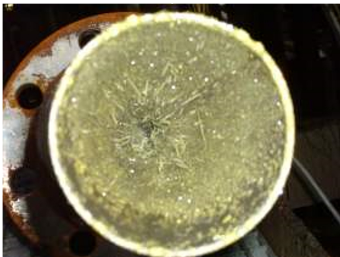
Figure 3: Buildup on free space radar antenna, which does influence the safety function.
