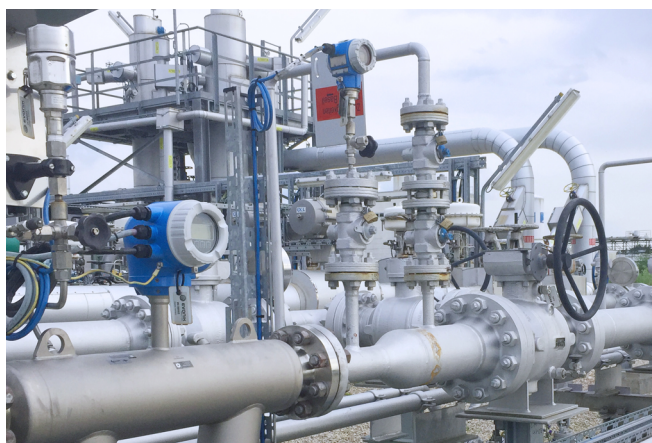
Figure 1: Flowmeters like those shown here can play key roles in reducing risk with safety instrumented systems (SIS).
