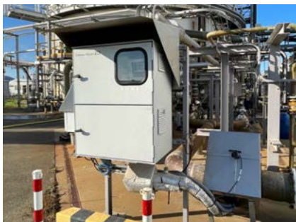
Automated wastewater monitoring: CDC90 with weatherproof cabinet and heated insulating cap for fitting and sensor
